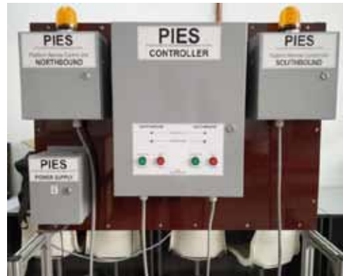
Local control panel installed at the railway station's equipment room
