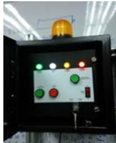
Platform control panel
